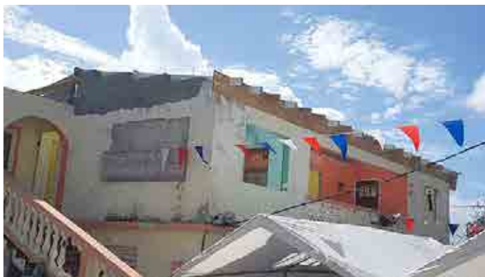
A second house in the French Quarter is in the process of being repaired.
