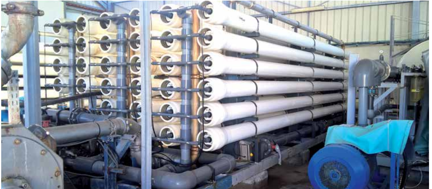
Reverse osmosis water desalination system
